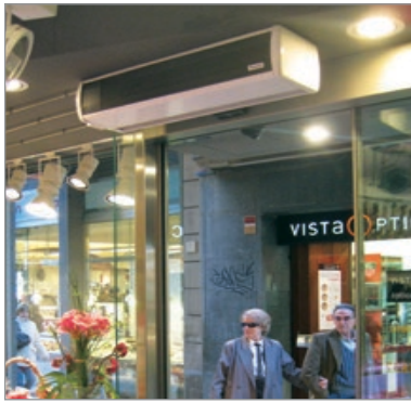
Optima Installation in a shopping center
